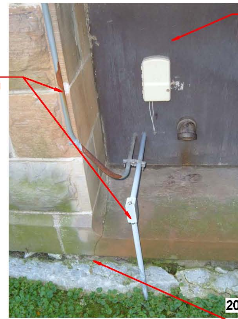
20 REMOVE PLYWOOD PANEL, INSTALL NEW TREATED PLYWOOD PANEL w/ PRE-FINISHED METAL WALL PANEL w/ SELF-ADHERING SHEET WATERPROOFING, SEAL AROUND PERIMETER OF PRE-FINISHED METAL WALL PANEL. (EXTERIOR SHEET METAL PACKAGE)
