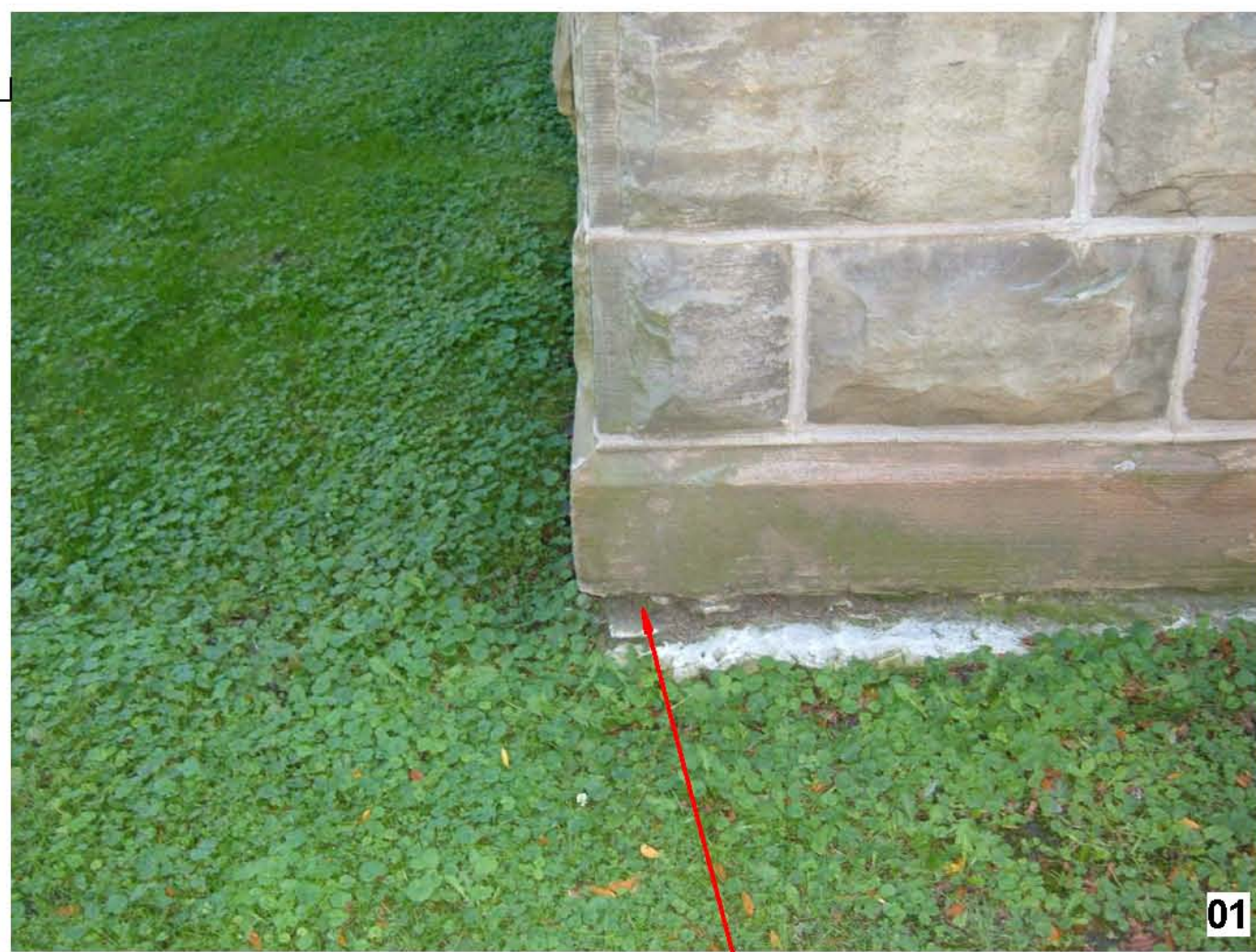
REPAIR JOINT @ FOUNDATION - REMOVE LOOSE MORTAR, TUCKPOINT W/ MORTAR, TYPICAL FOR PERIMETER OF BUILDING.
