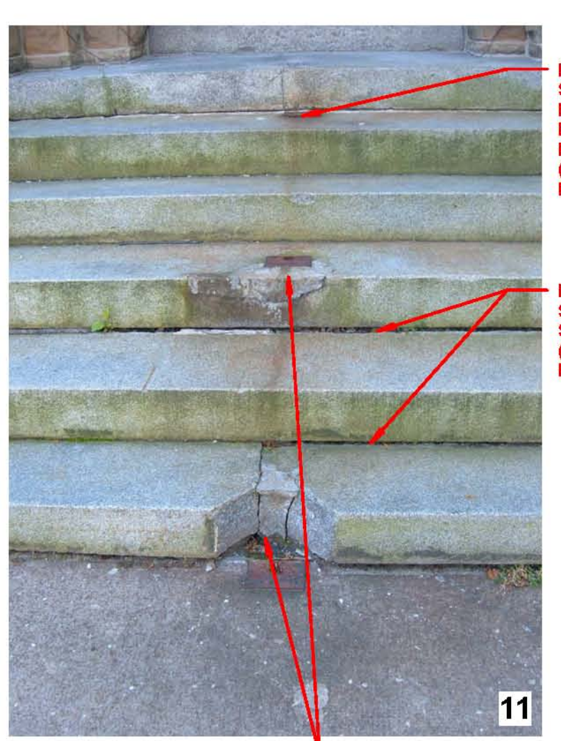
INSTALL NEW GALVANIZED STEEL PIPE HANDRAIL, MATCH EXISTING RAILING DESIGN ON EAST STAIR, PAINT. (STONE RESTORATION PACKAGE) INSTALL BACKER ROD & SEALANT, TYPICAL @ ALL STEPS (STONE RESTORATION PACKAGE)
