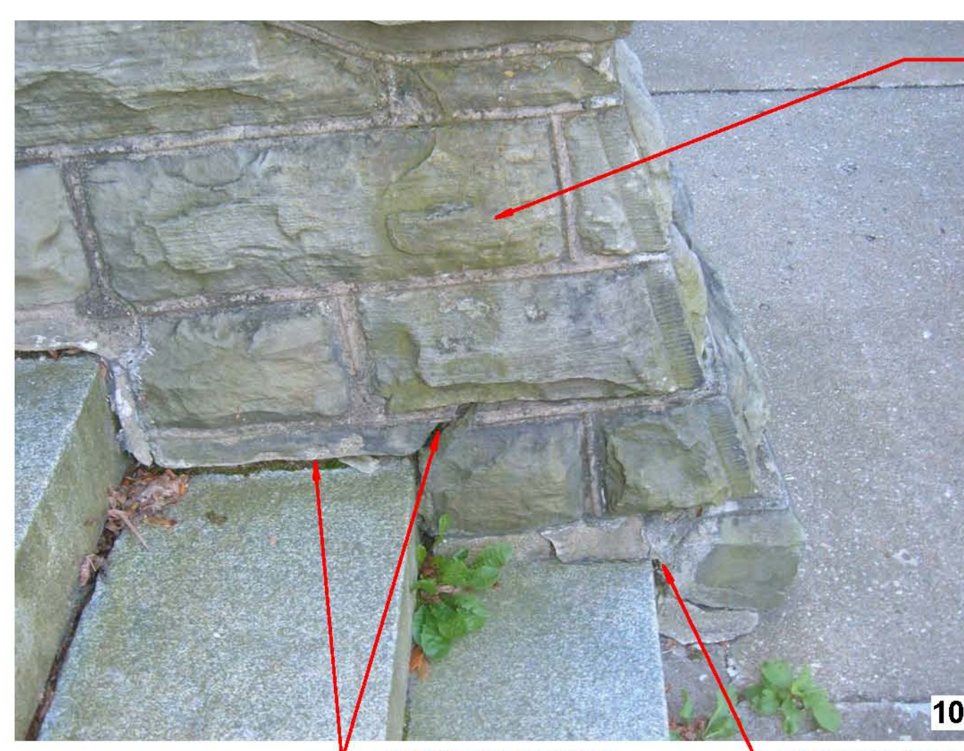
REMOVE MORTAR, INSTALL BACKER ROD & SEALANT. (STONE RESTORATION PACKAGE) REPAIR STAIR WALL (STONE RESTORATION PACKAGE)
